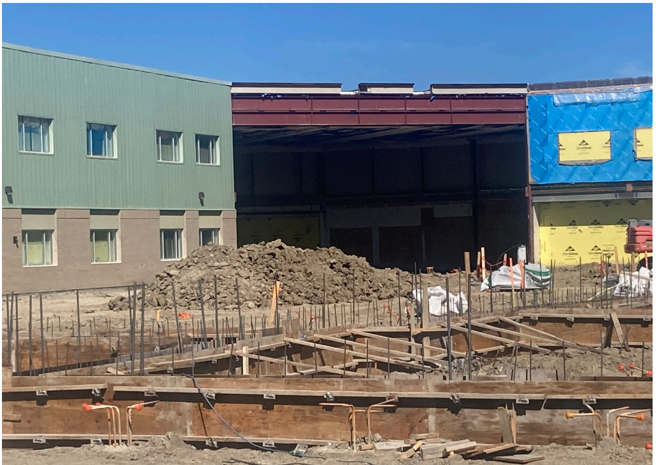
Construction to expand and modernize Bow Valley High School in Cochrane began in the spring of 2024.
